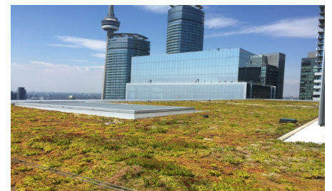
During long dry periods, an integrated irrigation system provides the vegetation with water.
